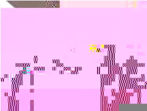
Sagging ceiling grid and tiles in office
