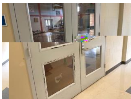
Gym steel doors needs repair
