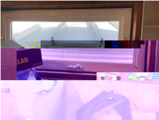
Mildew on window seal
