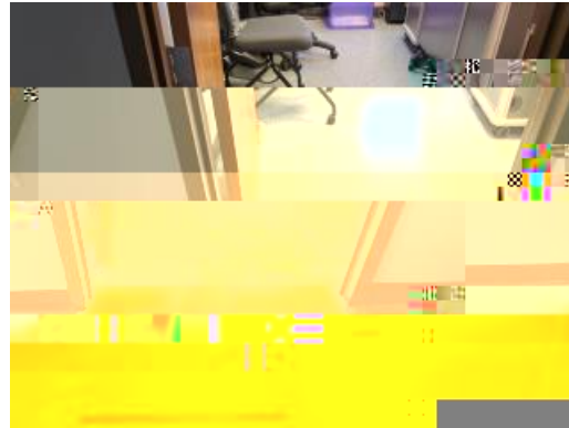
Damaged epoxy floor
