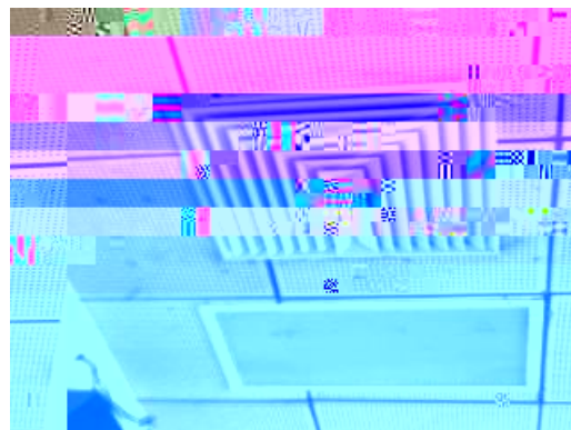
Damaged ceiling tiles
