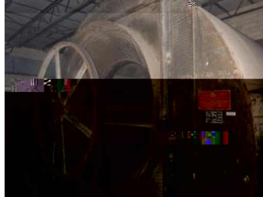
Aged and rusted supply fan
