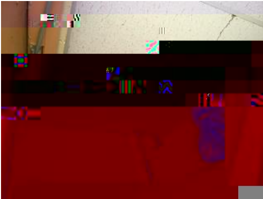
Broken acoustical ceiling tile
