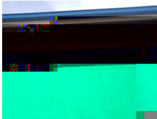
Damaged exterior insulation finishing system
