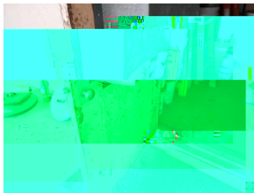
Damaged exterior metal door
