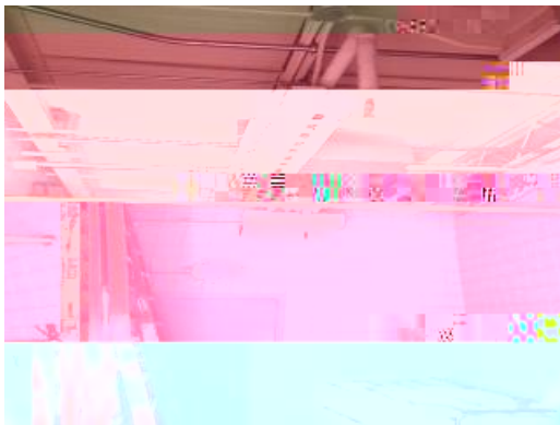
Deficient interior lighting
