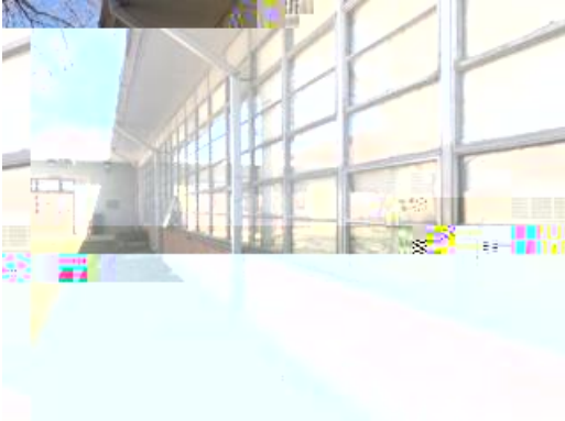
Exterior windows beyond service life
