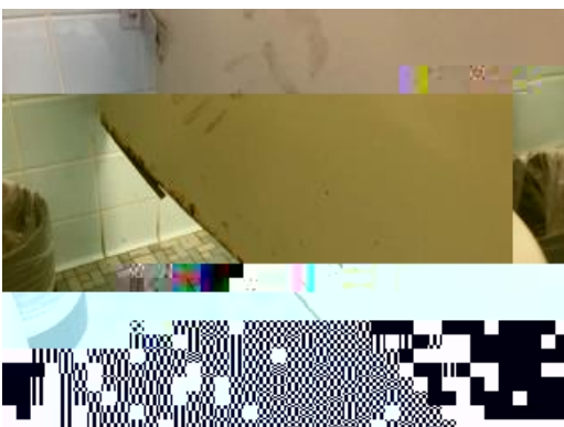
Aged toilet partitions
