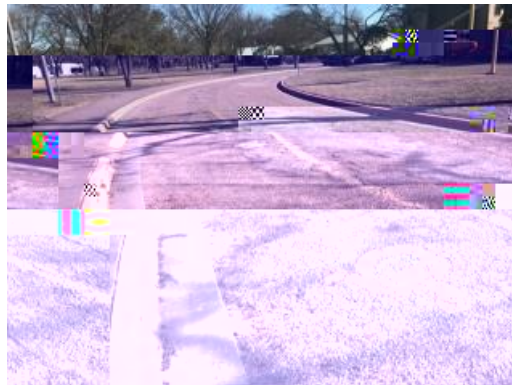
Asphalt drive past useful life
