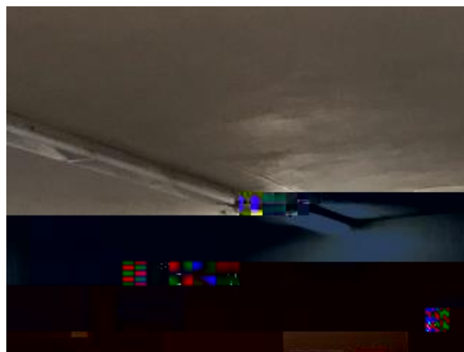
Warped plaster ceiling
