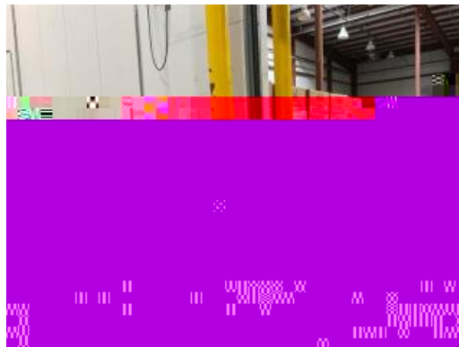
Damaged insulated sliding door
