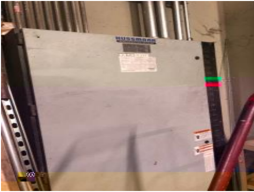
Hassmann panel inaccessible
