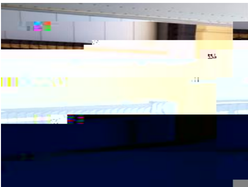
Damaged wall panels
