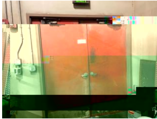
Steel doors are beyond their useful life
