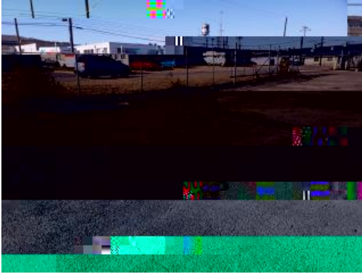
Asphalt pavement at end of life
