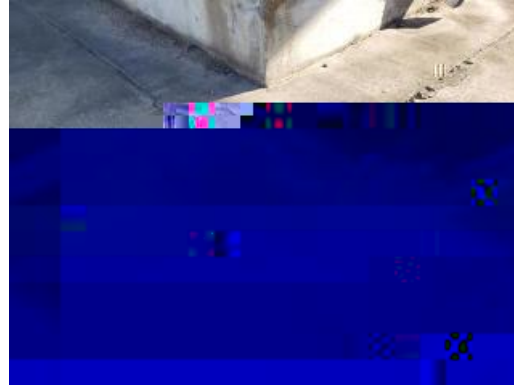
Cracked concrete pavement.
