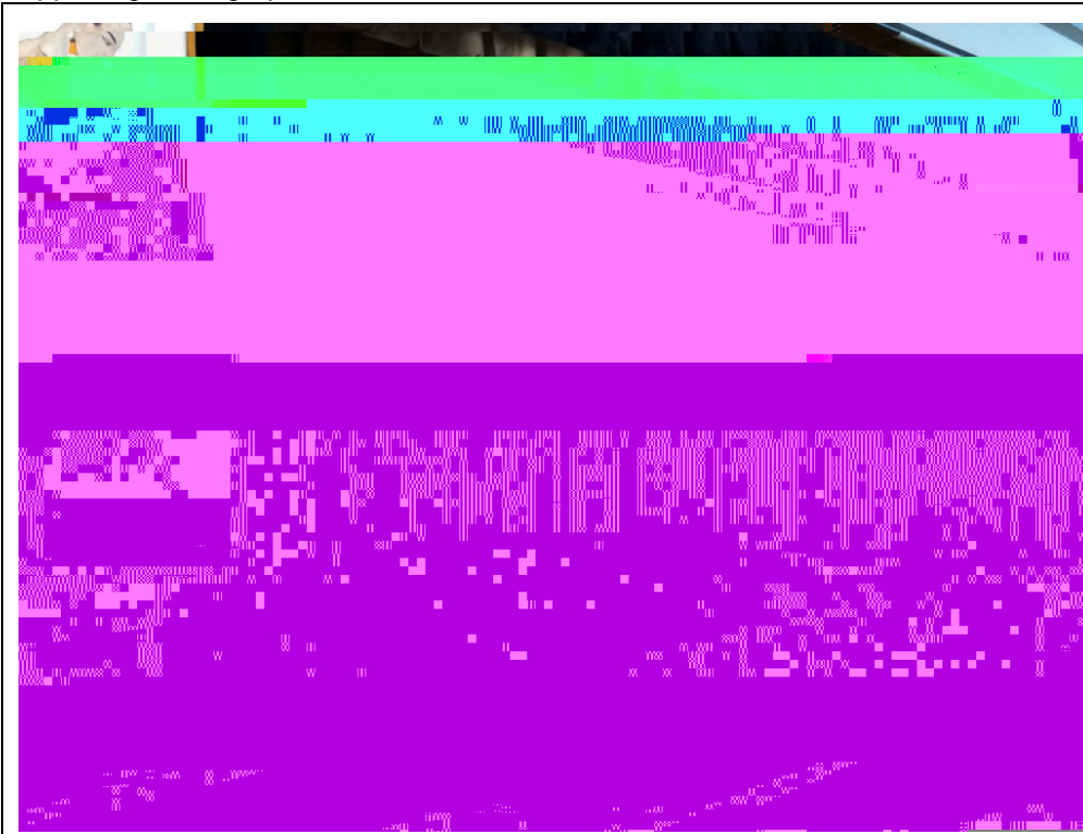
Visual and Performing Arts: Cafeteria stage needs updates, including lighting, audio system, flooring and curtains. A lift is provided for accessibility.
